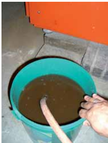
Heating water sample 09.05.2008
